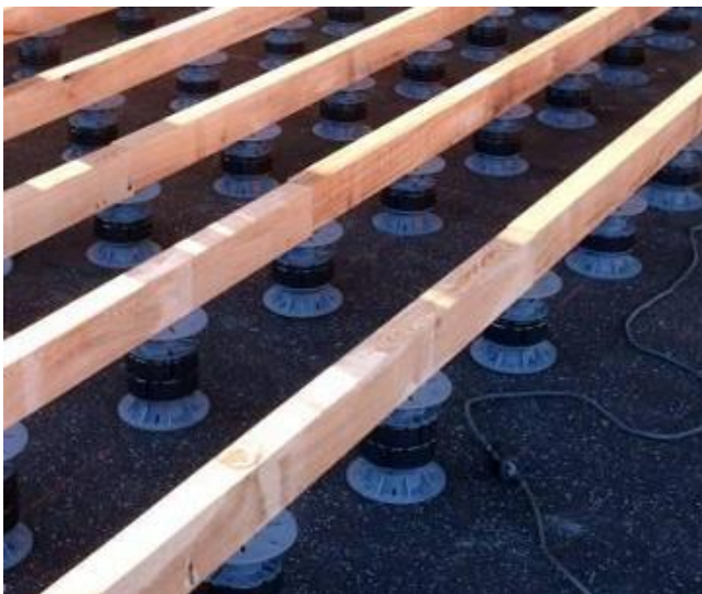
Fig. 5: 2 PP155/45 stacked between 2 PLV 50/75, Project MPI Tübingen.
